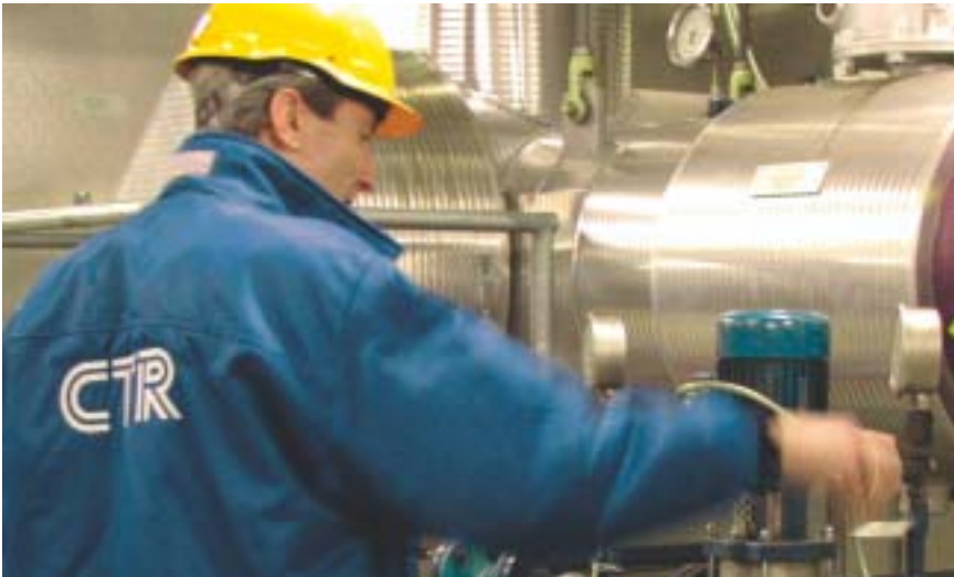
An exceptionally detailed regulation of the temperature of the system can lead to appreciably large savings
