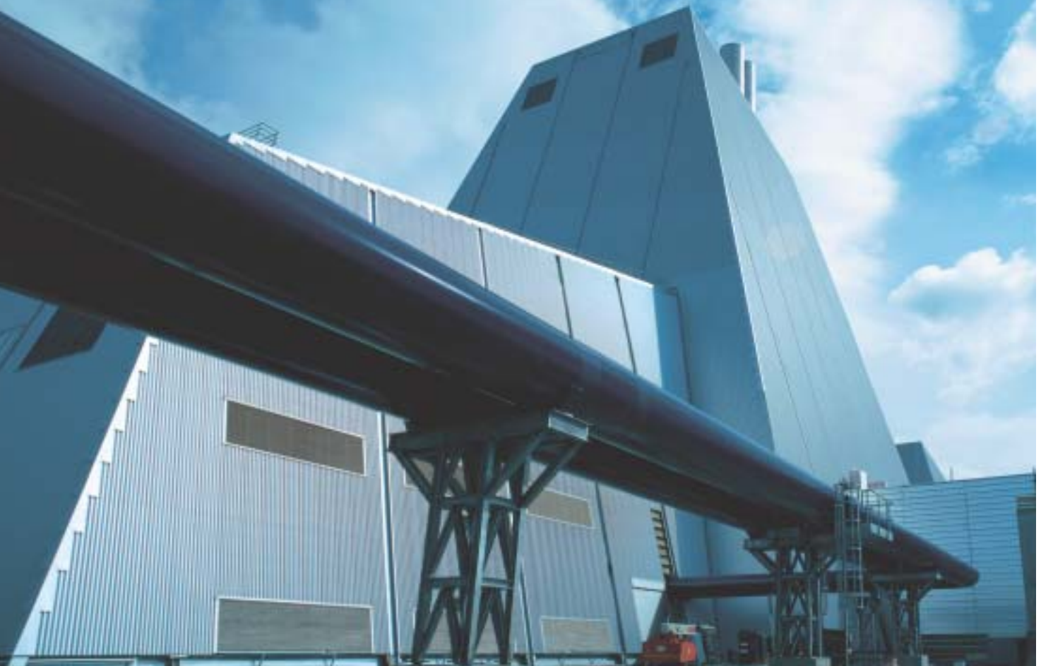
Transmission, steel-in-steel pipes leaving Avedore plant
