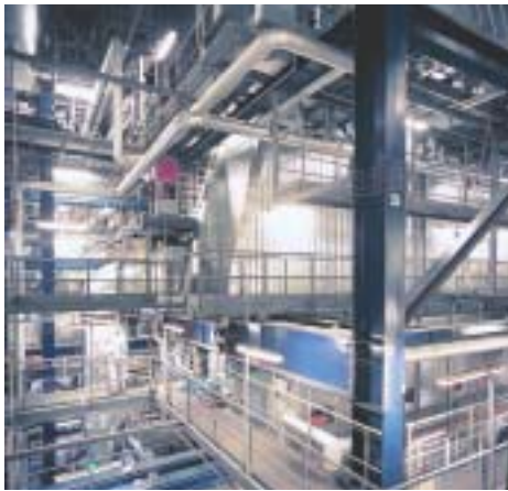
Part of Avedøre 2 plant
