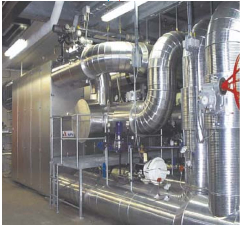
The 26 heat exchangers is the dividing line between CTR and the municipal companies
